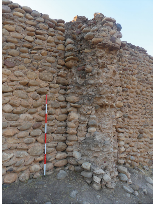
Figure 13 Interruption of the banks for the construction of the tower (western external wall)
